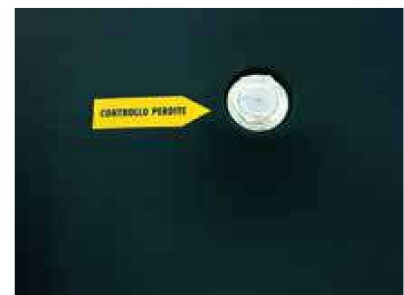
Monitoring light in the interspace
